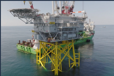
ELECTRONIC SERVICE PLATFORM (OFFSHORE SUBSTATION)
